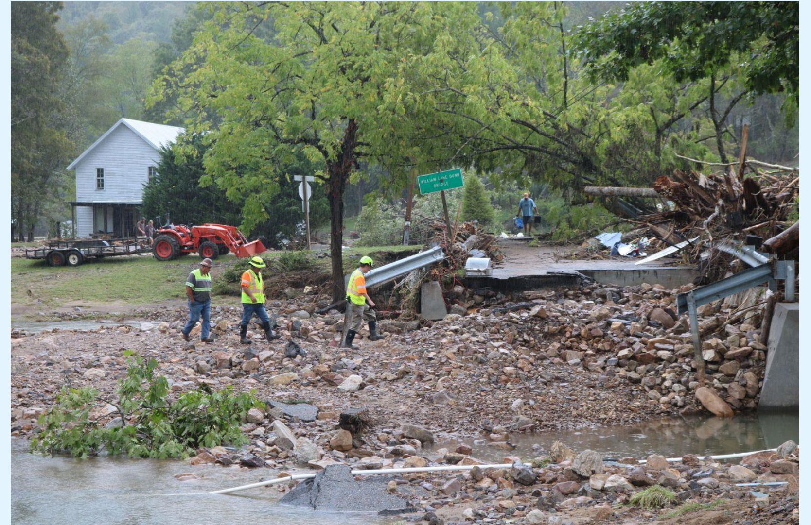
Following the remnants of Hurricane Helene, the Virginia Department of Transportation's (VDOT) Bristol District has worked diligently to re-open roads and remove debris. https://www.vdot.virginia.gov/news-events/news/bristol-district/hurricane-helene-roadway-recovery-efforts-continue-in-southwest-virginia.html
